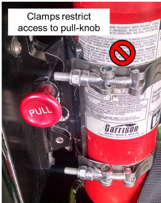
Figure B-51: Incorrect orientation of extinguisher clamps.
